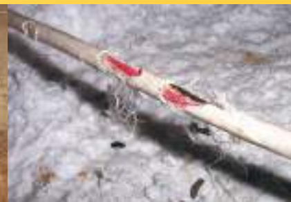
Gnawed Electrical Wiring
