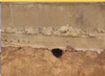
Foundation Burrowing & Damage
